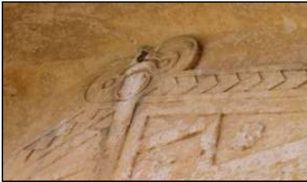
Figure 20. Loss of texture with salt formation on the unfinished monument
