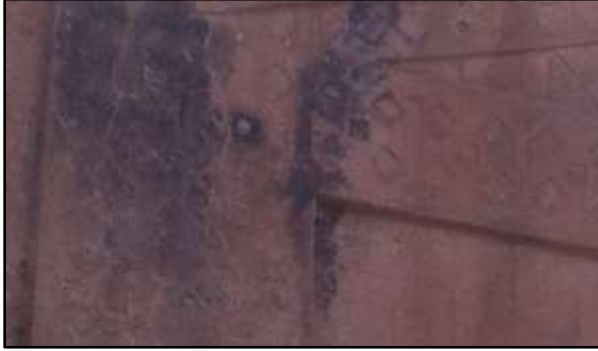
Figure 12. Black contamination and substance accumulation observed on Midas monument
