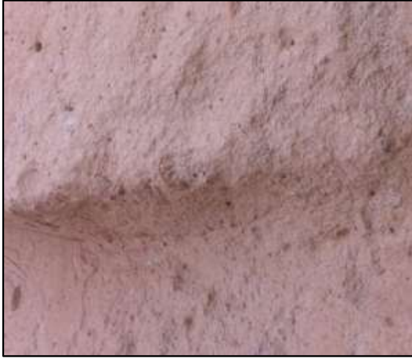
Figure 10. Loss of material with the type of sandblasting observed in Midas monument with the effect of rain and wind
